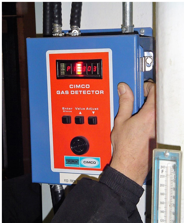
Figure 4 – Control Panel for Ammonia Leak Detection System
