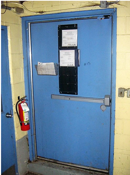
Figure 2 – Inside Door of Class T Machinery Room
