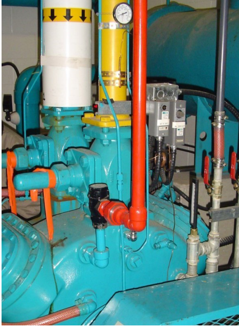
Figure 7 – Compressor Safety Valve
