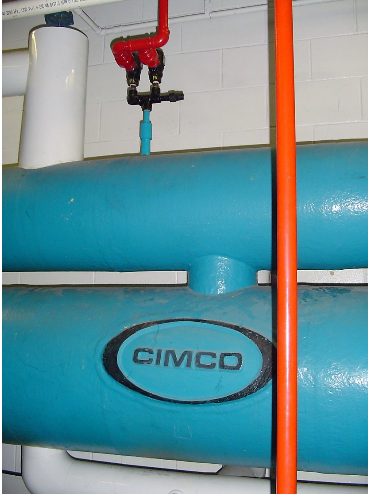
Figure 16 – Flooded Chiller with Surge Drum Mounted on Top
