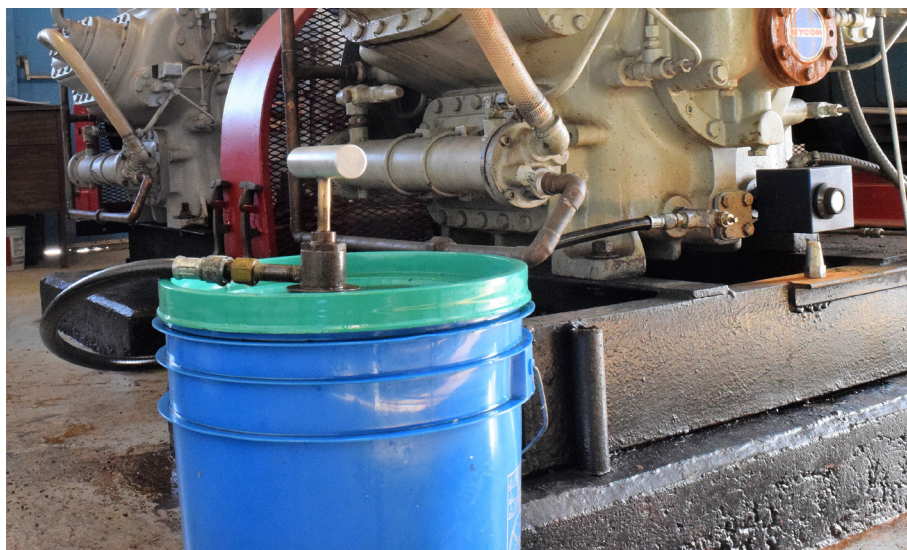
Figure 29 – Oil Charging Arrangement
