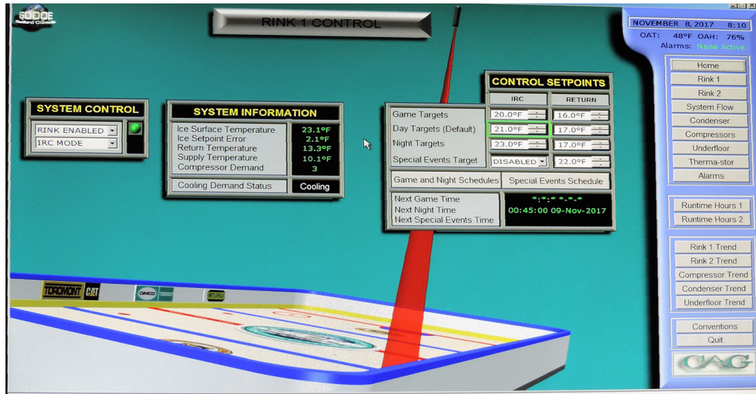
Figure 2 – Arena Ice-Making Equipment Control Screens
