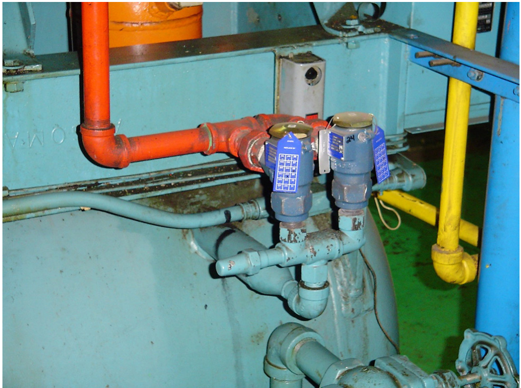
Figure 20 – Dual Safety Valve Installation
