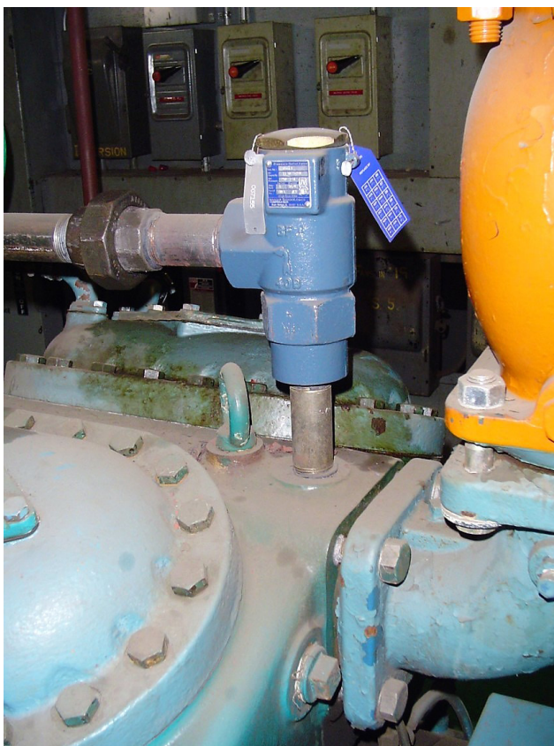
Figure 21 – Safety Valve for Positive-Displacement Compressor Protection
