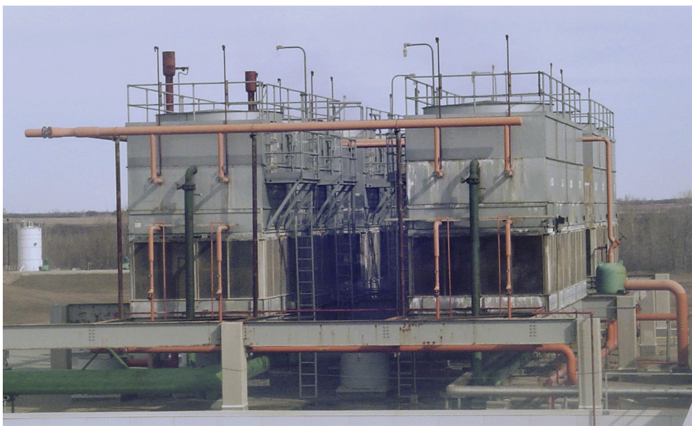
Figure 24 – Large Industrial Evaporative Condenser
