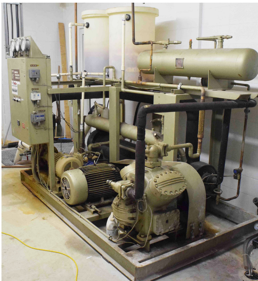
Figure 3 – Ice Rink Packaged Plant
