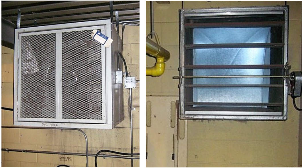
Figure 3 – Ventilation Fan and Exhaust Damper
