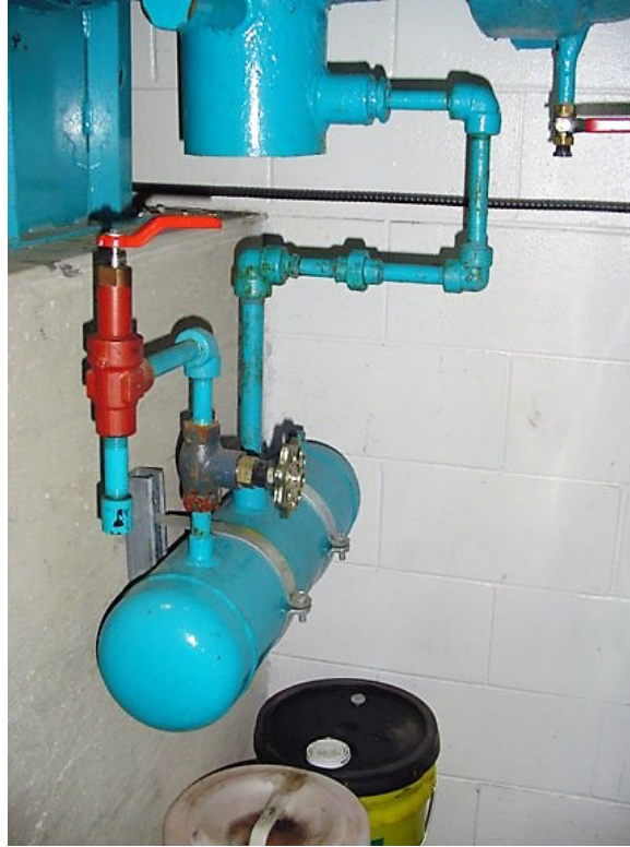
Figure 12 – Dead Man Valve for Draining Oil from a Refrigeration System
