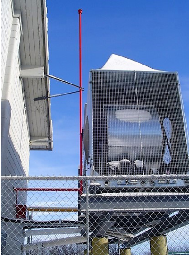
Figure 11 – Diffuser for Safety Relief and Emergency Discharge
