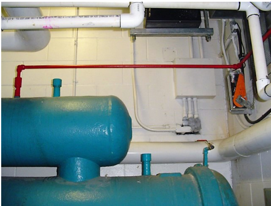
Figure 9 – Emergency Discharge Line Connection on a Chiller
