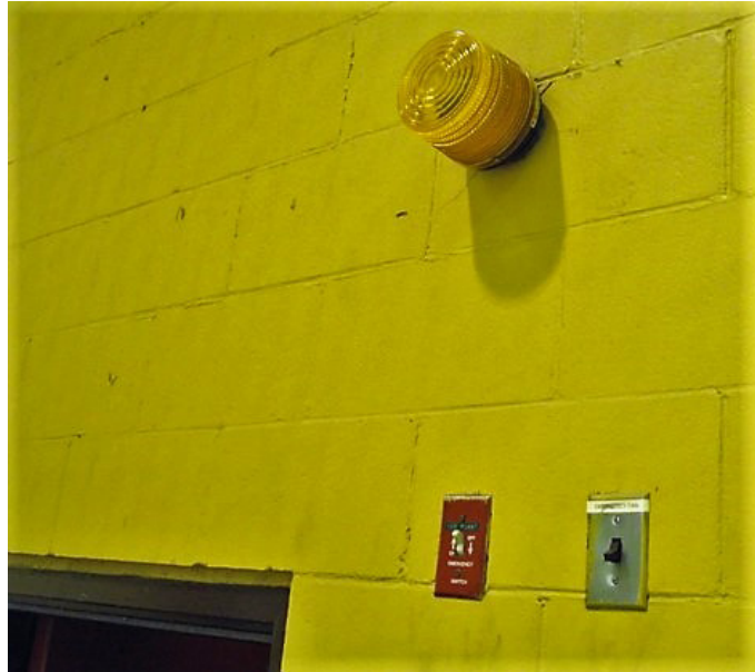
Figure 5 – Machinery Shutdown Switch, Ventilation Start Switch, and Alarm Beacon
