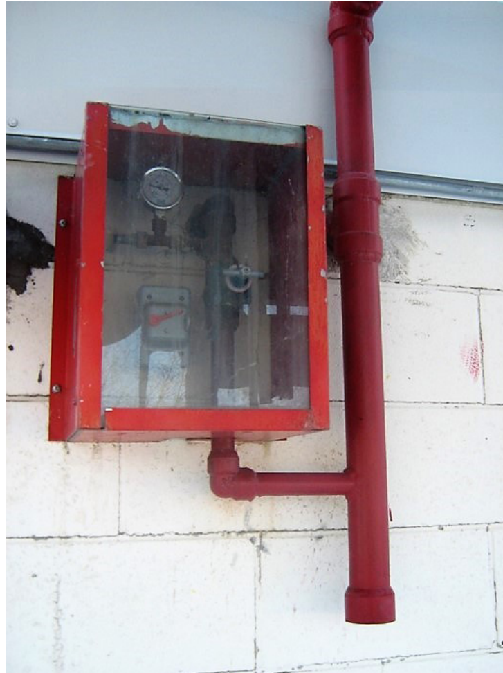
Figure 10 – Emergency Discharge Valve and Equipment Shutdown Switch
