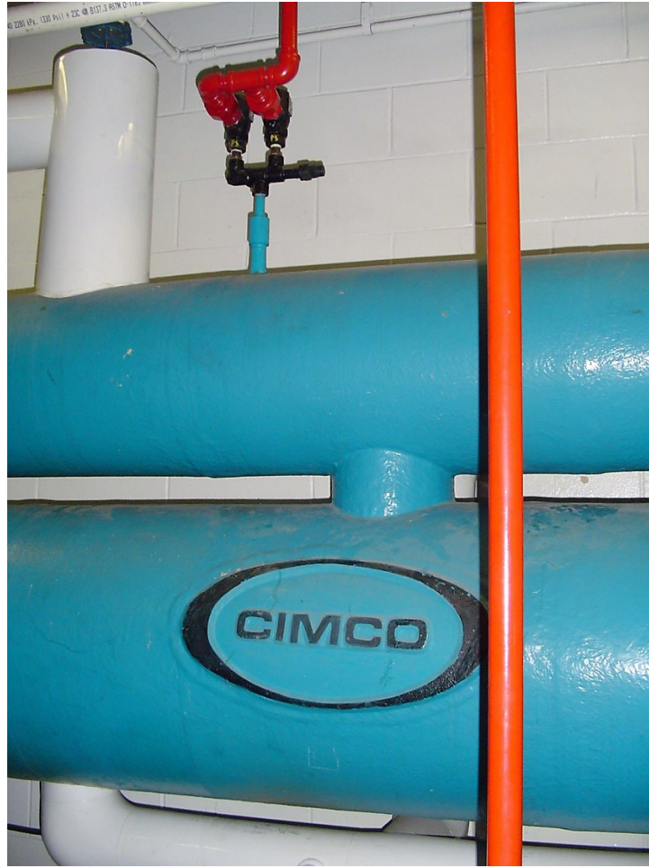
Figure 8 – Dual Safety Valves on a Chiller
