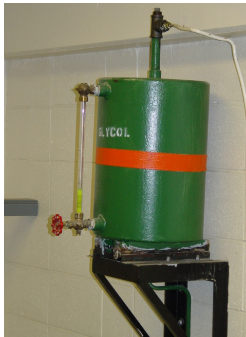
Figure 2 – Glycol Expansion Tank
