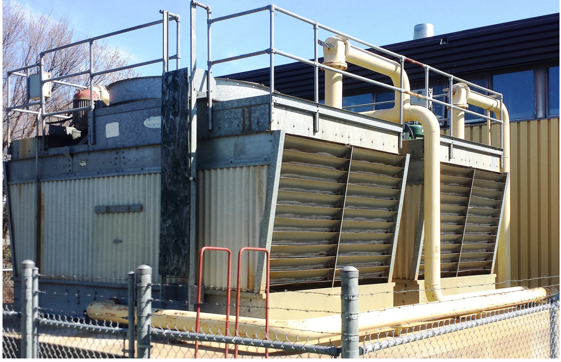
Figure 6 – Crossflow Cooling Tower in Service
