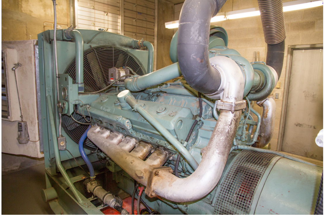
Figure 9 – Diesel Standby Generator
