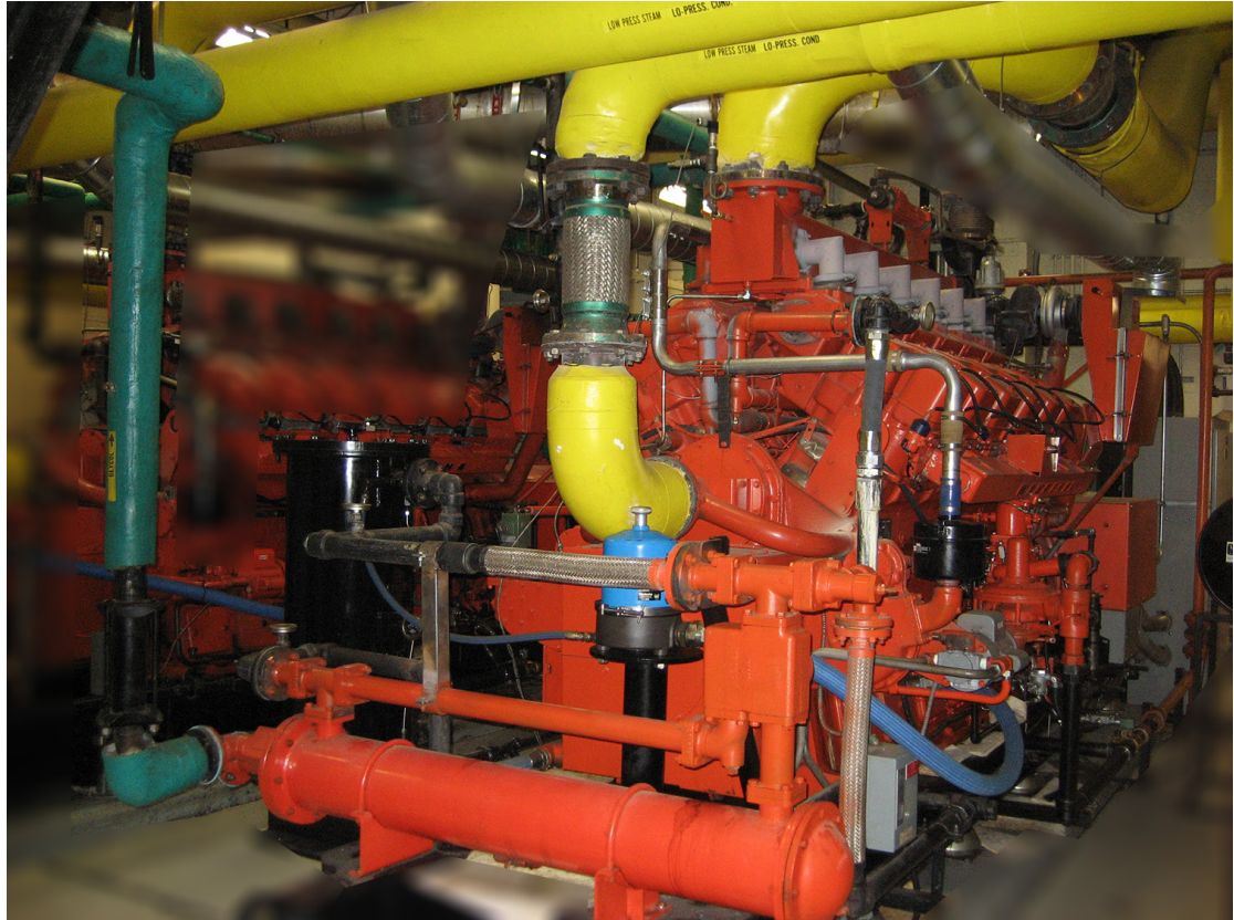
Figure 11 – Diesel Engine as part of a Cogeneration System
