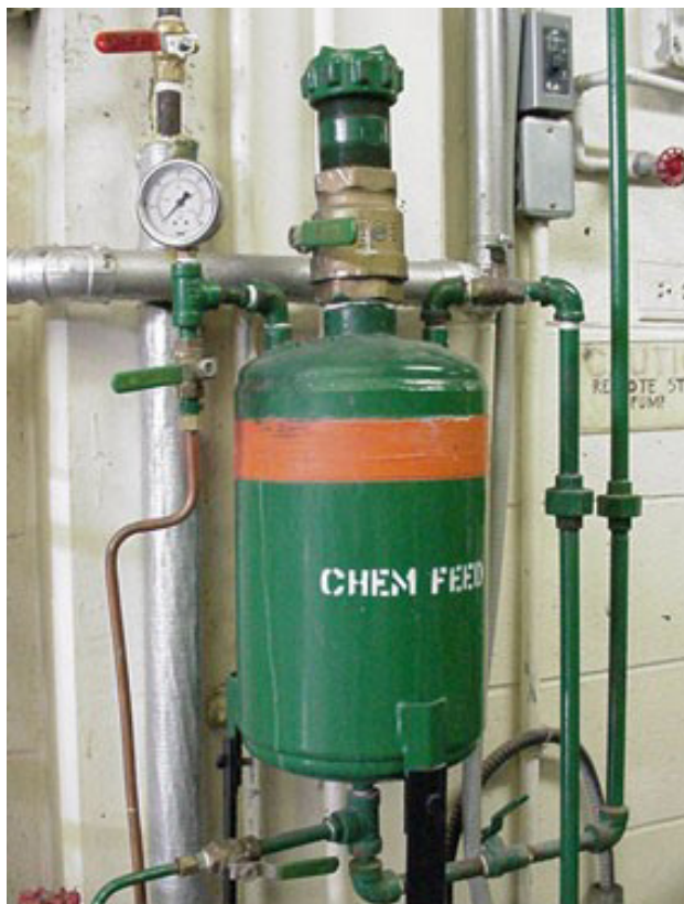
Figure 8 – Chemical Shot Feeder Installed
