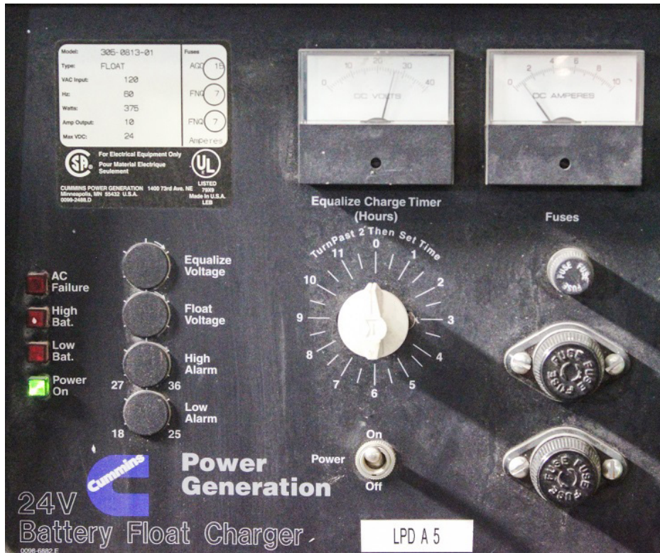
Figure 2 – Battery Charger for Diesel Standby Generator
