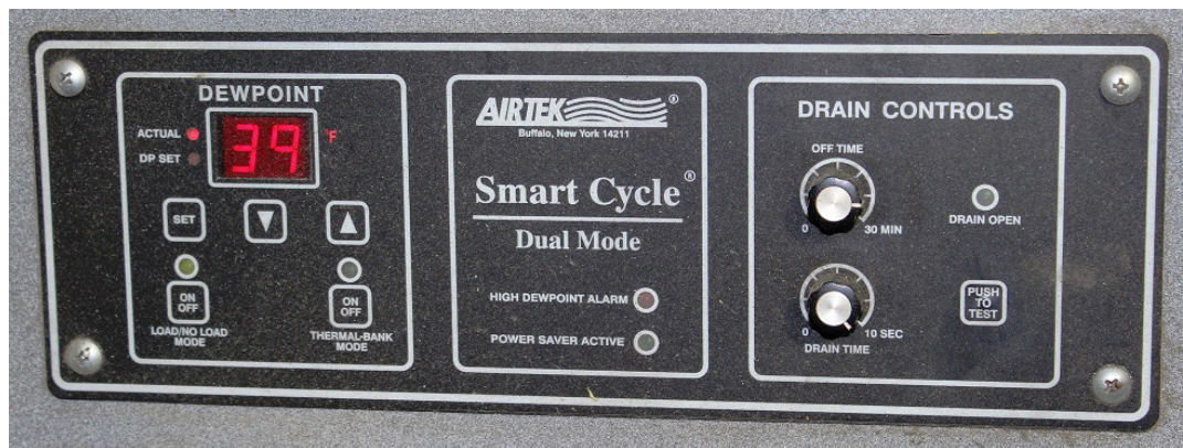
Figure 1 – HMI for Refrigerated Air Dryer, Showing Dewpoint
