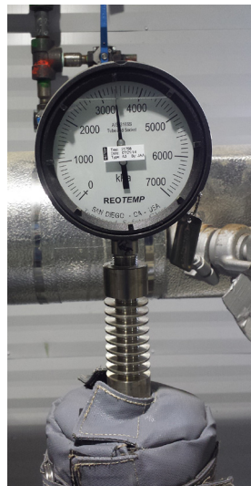
Figure 2 – Finned Siphon on a Steam Pressure Gauge
