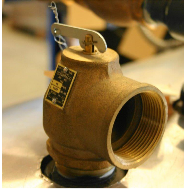
Figure 10 – Low-Pressure Safety Valve, Installed on a Steam Boiler
