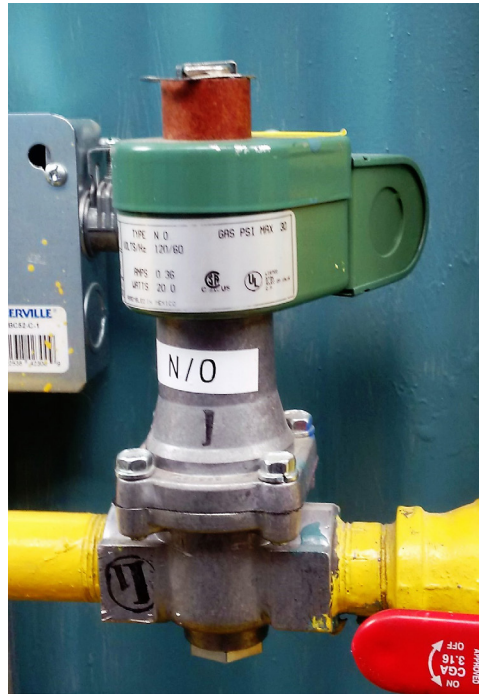
Figure 4 – Pilot Safety Vent Valve
