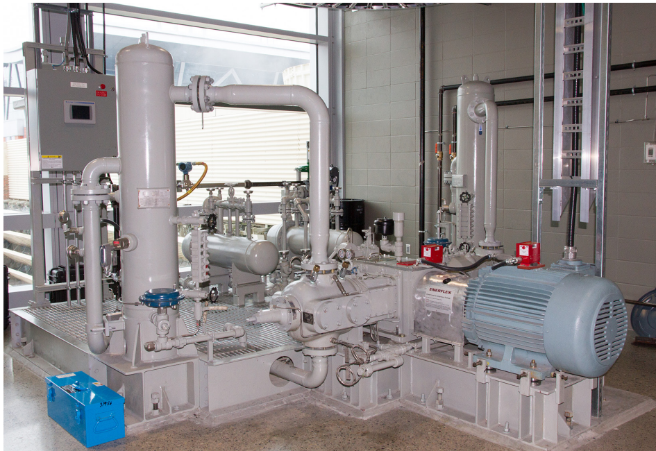
Figure 22 – Gas Compressor Skid Package
