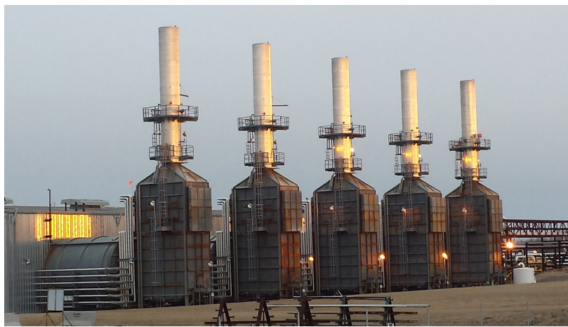
Figure 14 – SAGD Steam Plant
