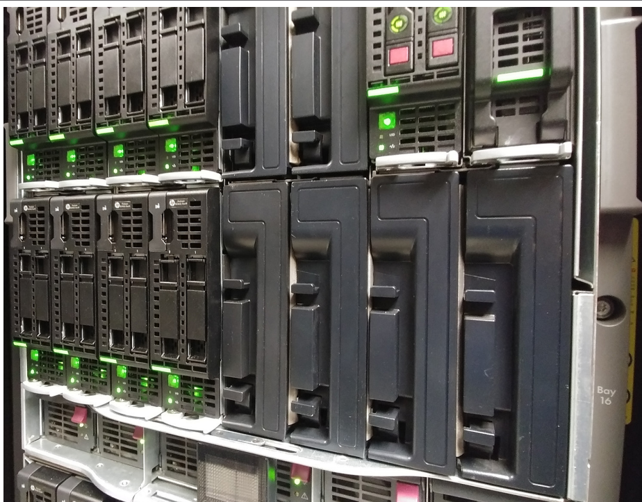
Figure 2 – View of a Server Room
