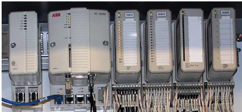
Figure 4 – ABB AC 800M Distributed Control System
