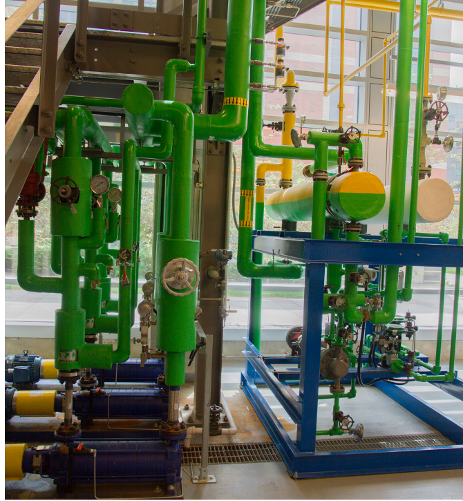
Figure 30 – Insulated Piping Systems
