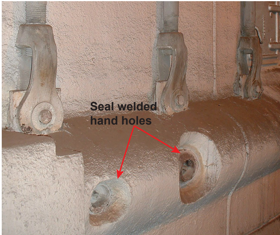
Figure 30 – Seal Welded Handhole in a Header
