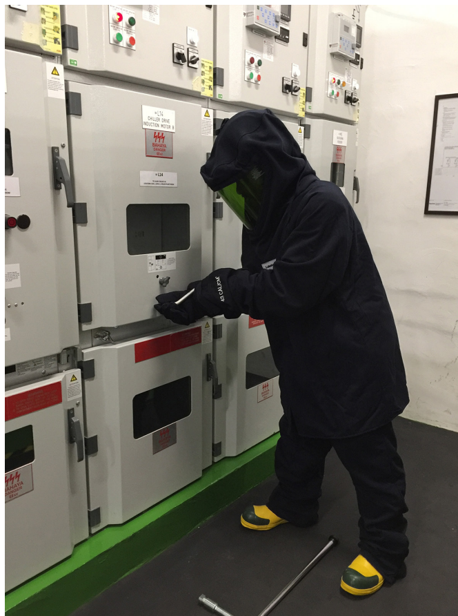
Figure 8 – Operating an Electrical Disconnect Switch with Arc Flash PPE
