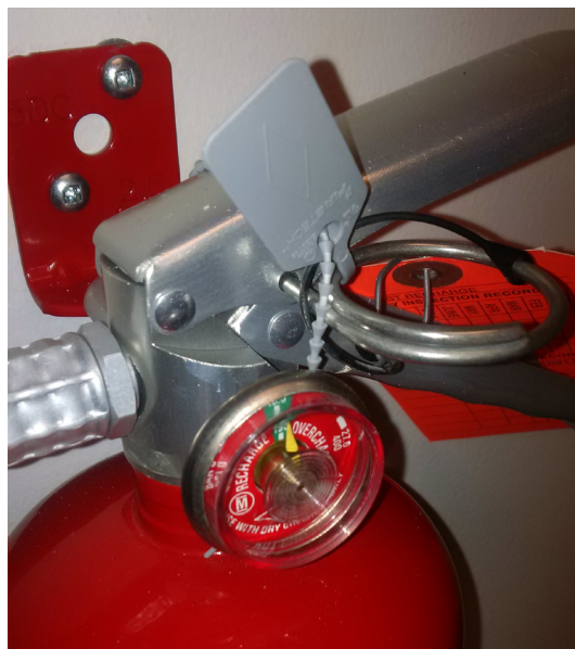
Figure 11 – Pressure Gauge and Seal on Extinguisher
