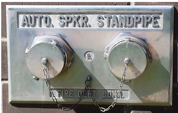
Figure 13 – Fire Department Connection
