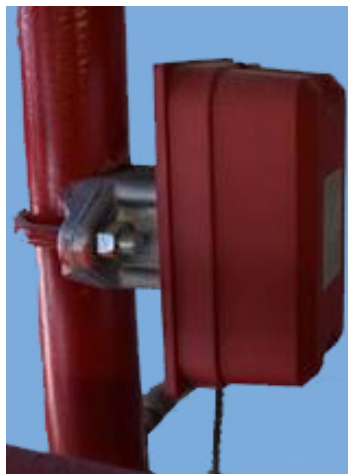
Figure 18 – Flow Switch in a Fire Line (Fire Main)
