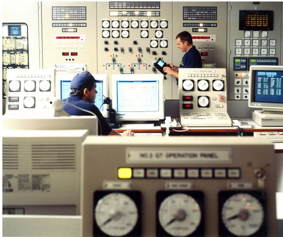
Figure 7 – Central Control Room
