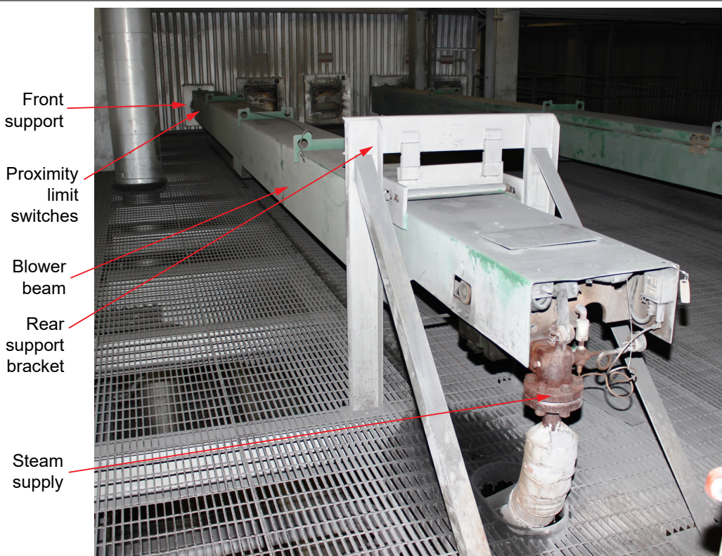
Figure 4 – Long Retractable Soot Blower
