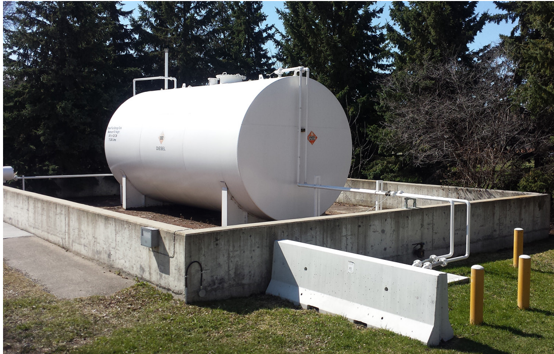
Figure 32 – Diesel Fuel Storage Tank Showing Supply and Return Lines
