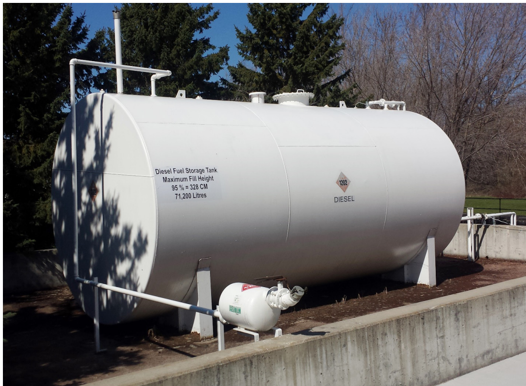
Figure 31 – Diesel Fuel Storage Tank Located in a Secondary Containment Berm
