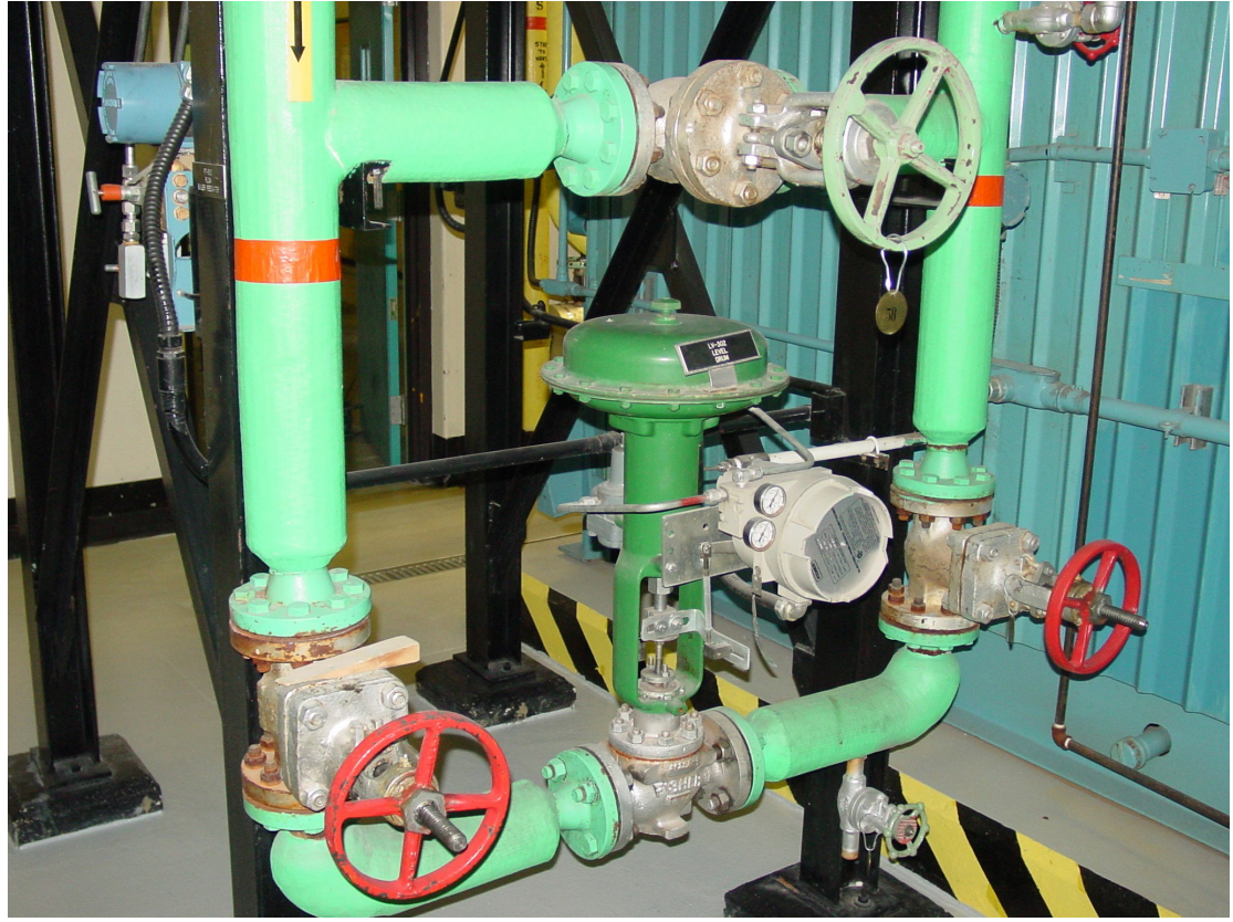
Figure 6 – Modulating Feedwater Control Valve Station
