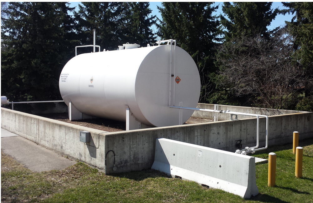
Figure 1 – Fuel Oil Tank with Containment Berm
