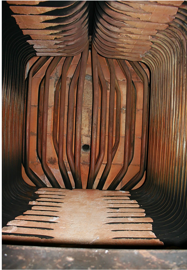
Figure 8 – Interior View of Watertube Furnace
