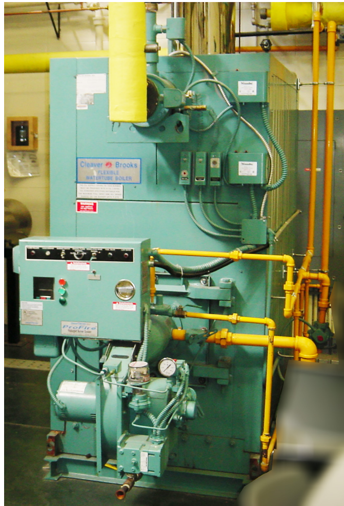
Figure 5 – Flexible Watertube Boiler in Heating Service
