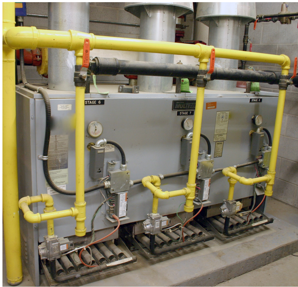
Figure 14 – Hot Water Plant with Multiple Boilers
