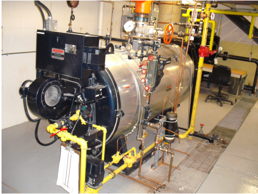
Figure 12 – Three-Pass Firetube Boiler
