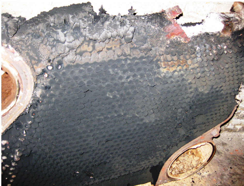
Figure 2 – Cast Iron Section Damaged by Poor Water Treatment
