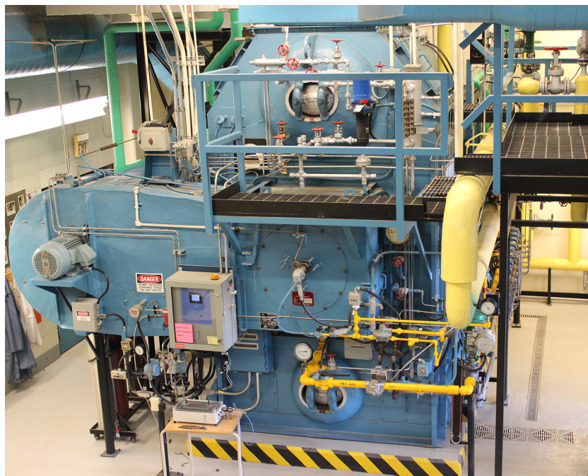
Figure 10 – Large Packaged Watertube Boiler
