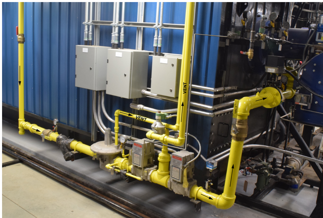
Figure 19 – Boiler Gas Train
